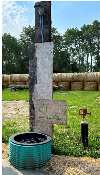
Drilled well and solar pump in yard.
