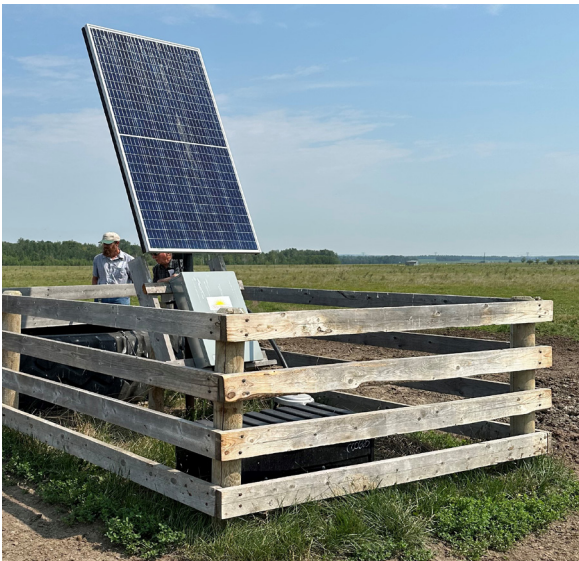
Drilled well and drain back winter watering system within a pasture.
